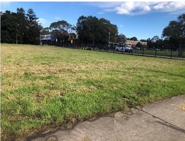
Photo 3 – Gas well BH1 likely damaged from lawn maintenance.
